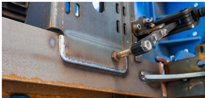
The seams welded by the robot produce a high weld seam quality and extremely low weld spatter, thus reducing post weld work by 30 per cent and increasing productivity.
